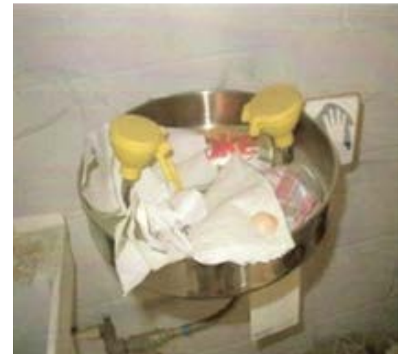
Example of an eyewash station that was not kept clear of debris nor tested weekly.
